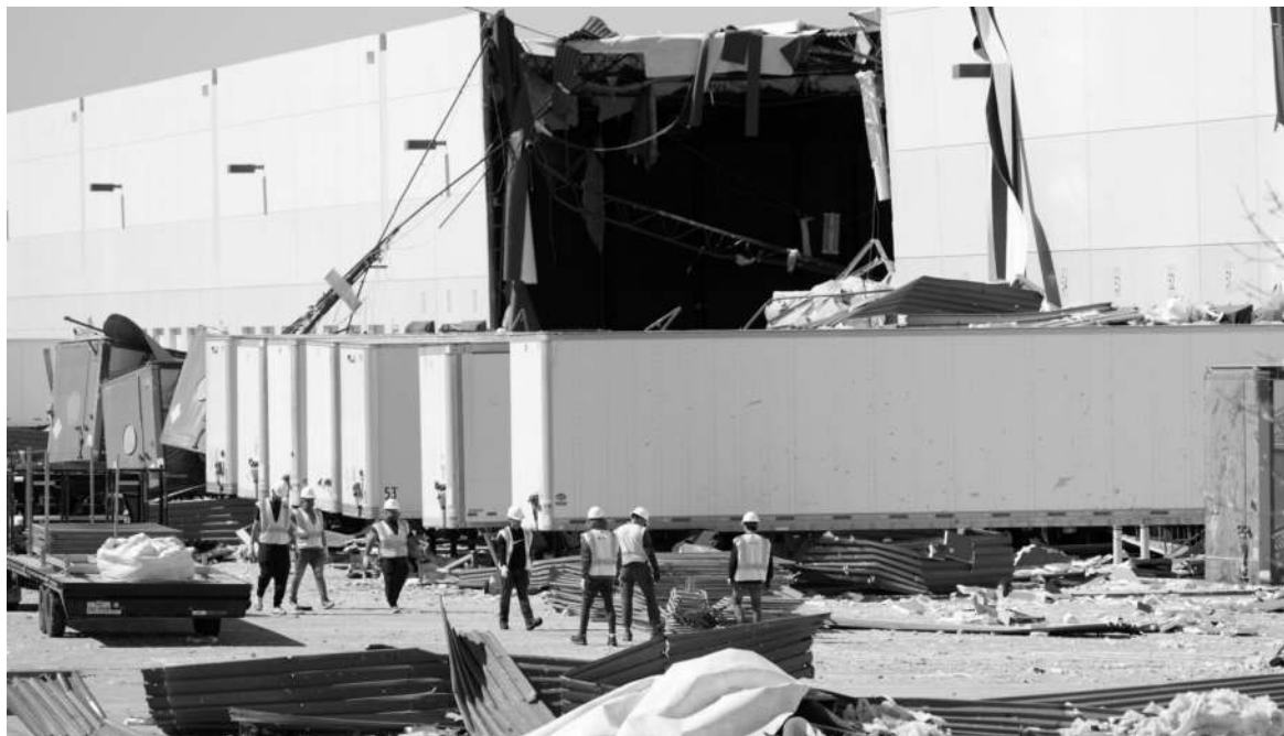
Workers walk outside a damaged warehouse after storms moved through Tuesday in Lewisville, Texas.
