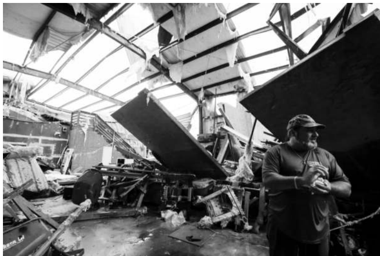
SCOTT THRELKELD, THE TIMES-PICAYUNE/THE NEW ORLEANS ADVOCATE/AP E.C.O. Builders' Lynn Champagne surveys damage after the building was struck by an apparent tornado in Slidell, La., on Wednesday.
