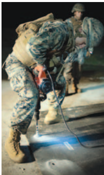
A combat engineer with Marine Wing Support Squadron 171 repairs airfield damage after a simulated missile strike during the Active Shield exercise Thursday at Marine Corps Air Station Iwakuni.
