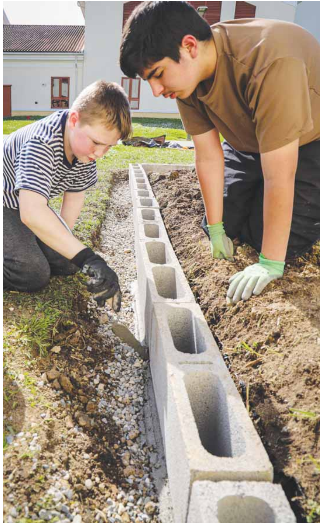
MARCELA ARTEAGA Max Arteaga, a 14-year-old Boy Scout, supervises a volunteer helping him lay a concrete block wall for his Eagle Scout project of restoring several decaying planter beds at the Department of Defense Education Activity elementary school in Vicenza, Italy.
