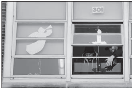
Workers on Thursday replace a window that was broken by gunfire at the Sacred Heart school during a gunbattle in Jersey City, N.J.
